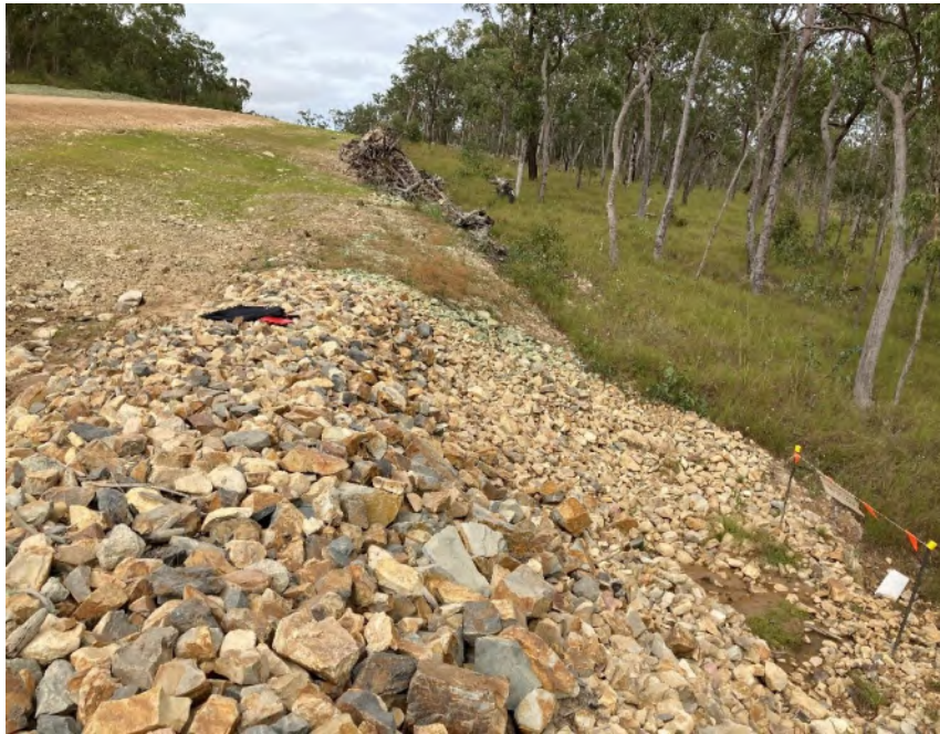
Topsoil re-instated after cable trenching along roadside. Rehabilitation underway as indicated by new grass shoots.
