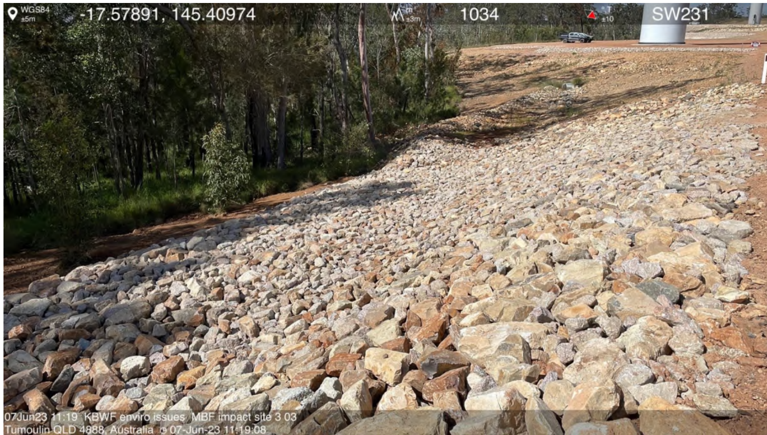
Rock-filled roadside drainage and huge sediment traps and level spreader to improve water discharge to magnificent brood frog habitat.
